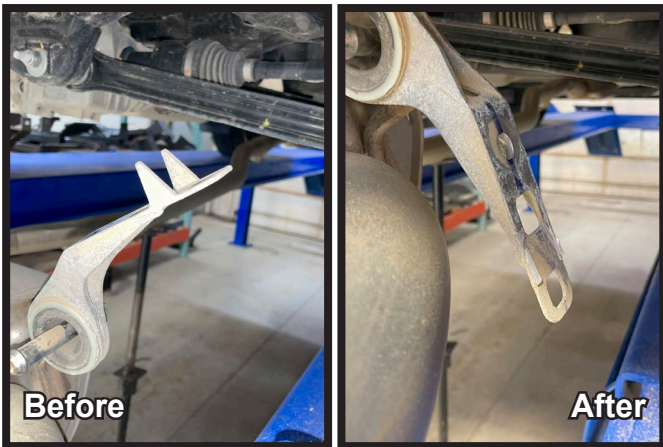
20a. Non-Trailhawk Models Only: Using a reciprocating saw, remove the triangle points from the exhaust bracket. Do this on both sides of the vehicle.
