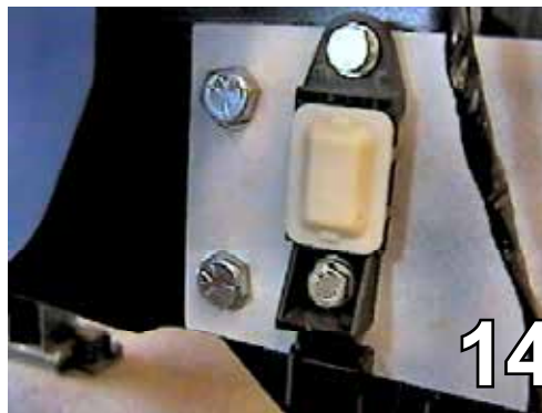
14. Using the diagonal cutters, cut off the alignment pin on the sensor and reinstall the sensor to its original position through obround holes on baseplate ends using the 6MM x 30MM hex bolts provided, both sides.
